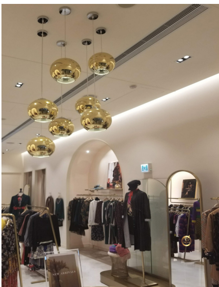
Application on a Retail Shop Installing in ceiling and working like a wallwasher, with SMD5050 led strips IP20, makes a soft light also with lighting control.
